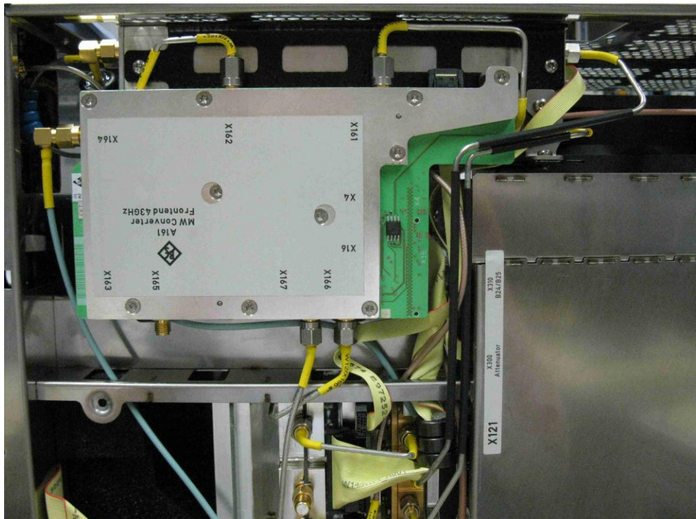
Figure 3-24: Cable routing on the lower side of an R&S FSW67 without option R&S FSW-B24 installed
